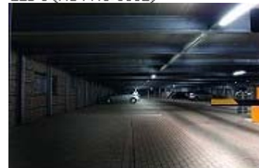
Basic night-time illumination with manual override wiring for individual lights
